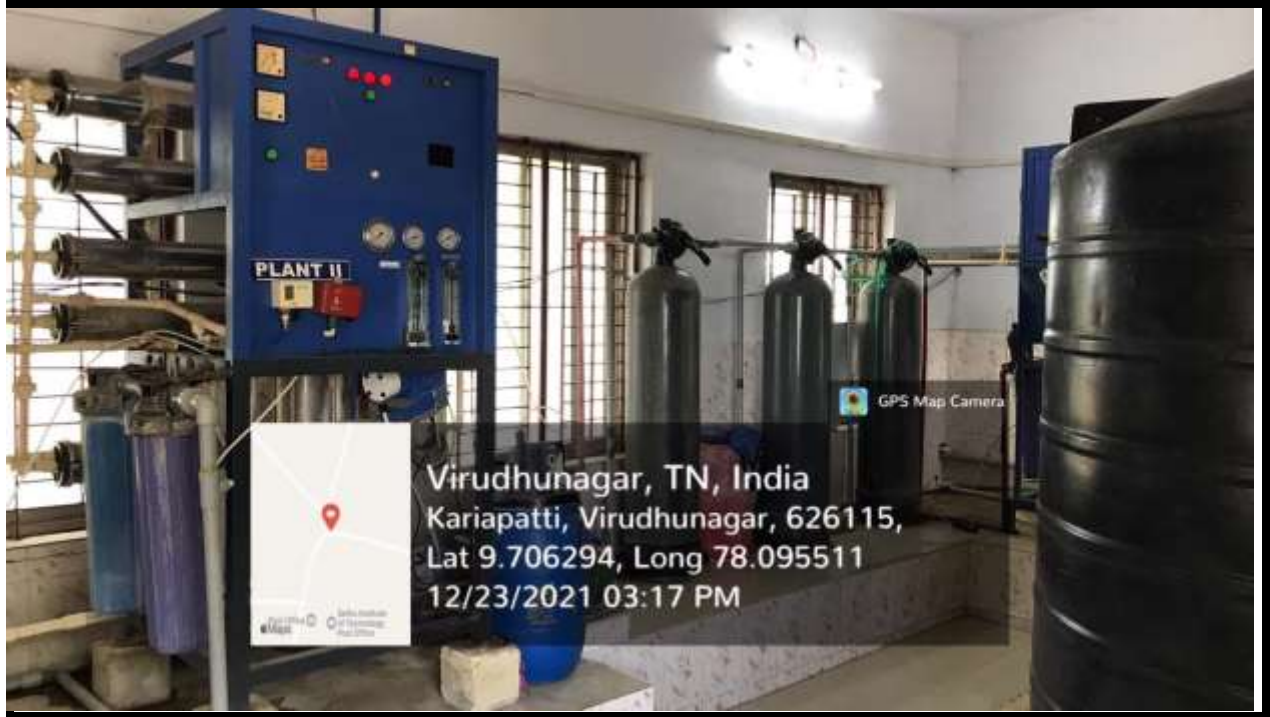
RO Water Plant
